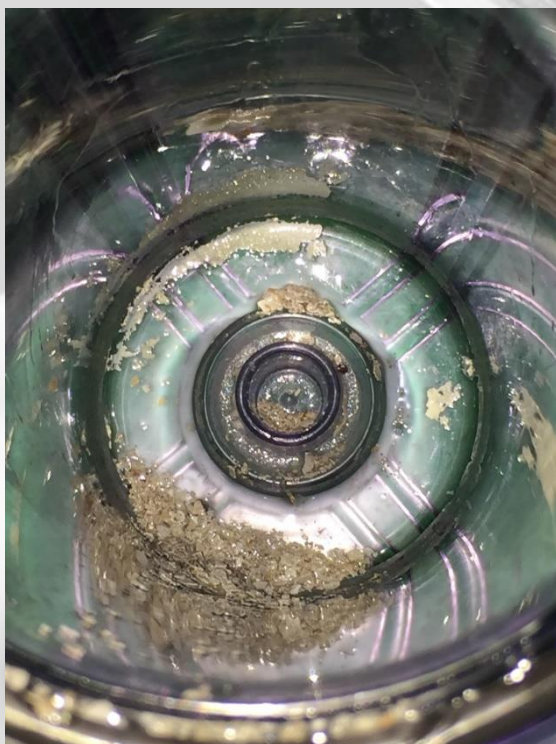
Calcium deposit in the filter jar after cleaning WSC系统过滤罐内水钙杂质
